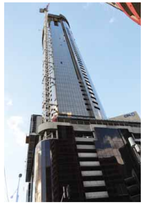
Prima Pearl is one of the new apartment towers being built to cope with Southbank's rapid population growth.
