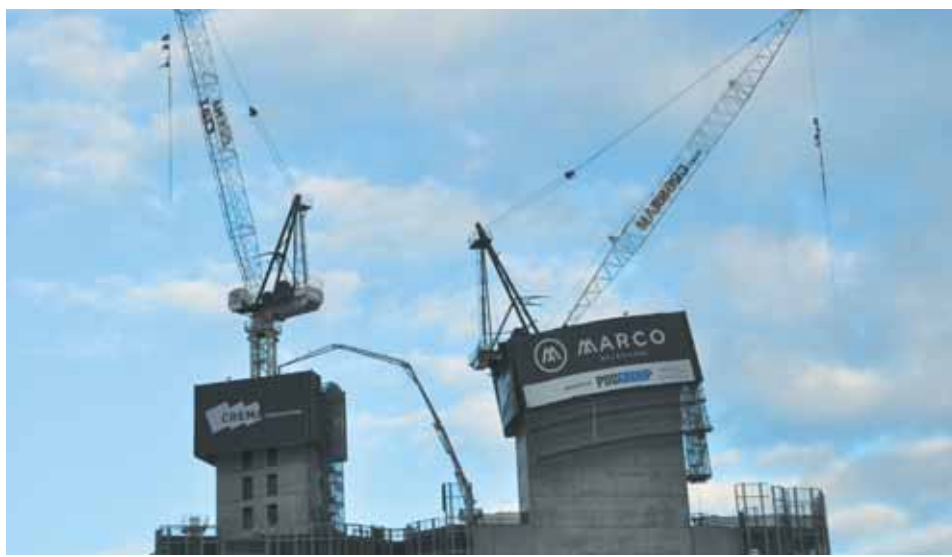
The crane at the construction site on Balston and Kavanagh Streets in Southbank, which was left resting on a lift shaft.
