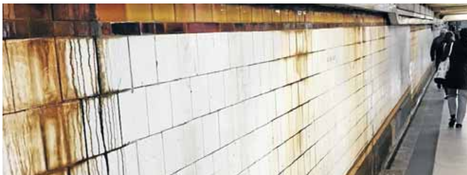
The run-down Flinders St underpass between Elizabeth St and Northbank.
