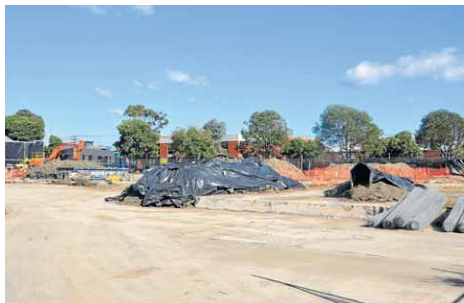
Works are underway at the site of the future primary school at Ferrars St.
