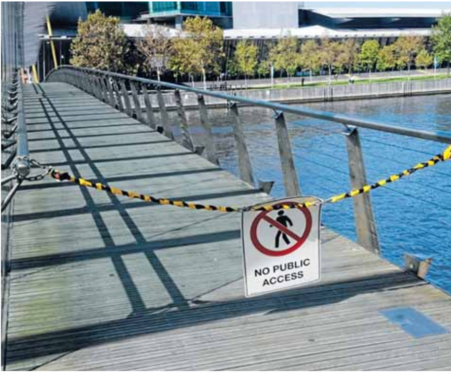
The walkway running along the Clarendon St Bridge has been closed for a considerable amount of time.
