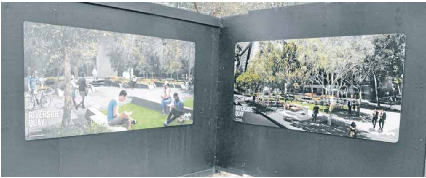
Renders of Mirvac's approved plans have appeared on the Riverside Quay renewal site's hoardings as construction begins.
