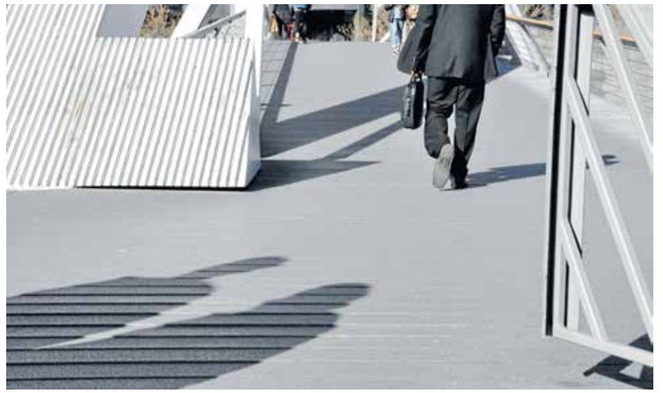
Loose decking on the northern end of the Evan Walker Bridge.
