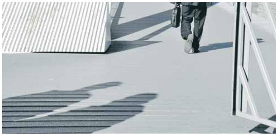
The loose decking on Evan Walker Bridge has resulted in increased noise over the past few years.
