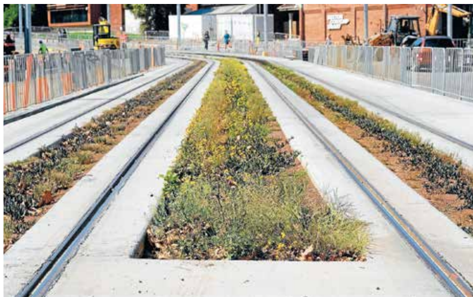
The new look tram tracks on Southbank Boulevard complete with new greenery, which was planted last month.
