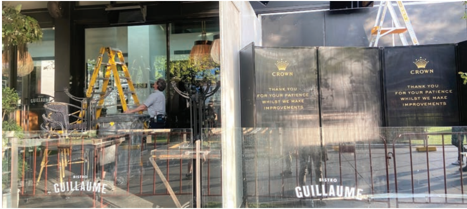
▲ Maintenance workers at Bistro Guillaume after fire caused damage to property.
