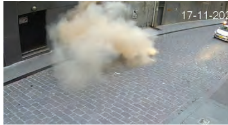
▲ CCTV footage captured a substation exploding after an attempted theft of copper.
