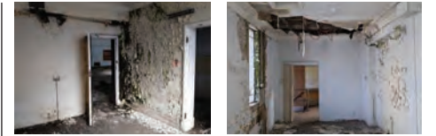
▲ Images showing the building's state of disrepair.
