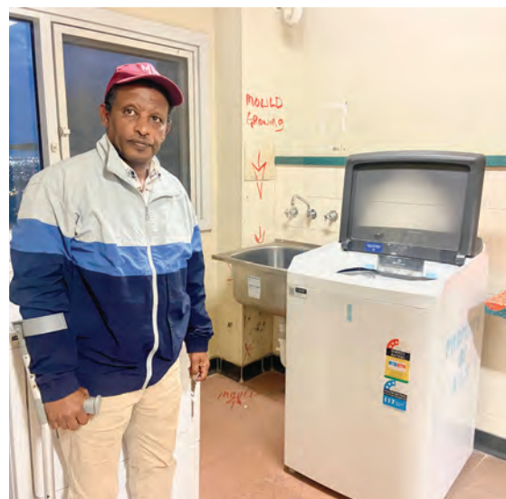
▲ Resident Mohammed Ahmed in the common laundry room where black mould has begun spreading.
